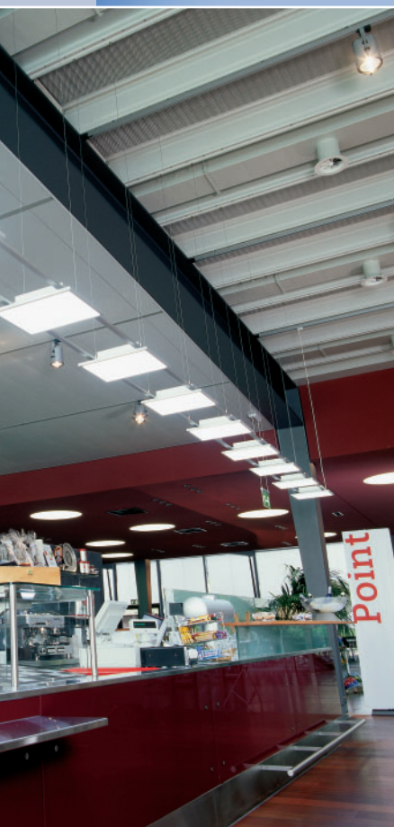
The Siemens Schweiz AG canteen – the soft, diffuse light of PLANON® provides virtually shadowless illumination.
